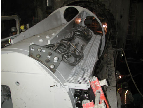
Figure 3 – Hyperbaric Chamber – Installation
